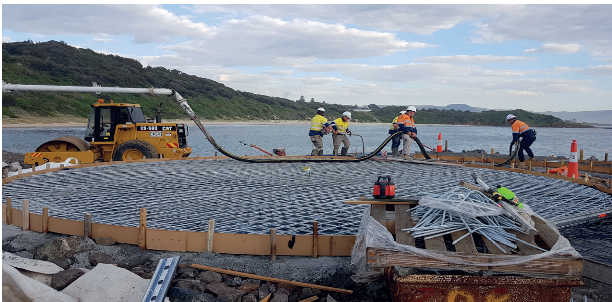
Image credit: Cleary Bros (Bombo) Pty Ltd – Red Point Rock Revetment, Port Kembla.
