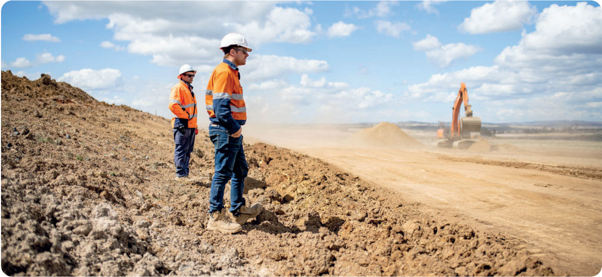
Image credit: Townes Contracting Group. Construction of New England Solar Farm, east of Uralla NSW.
